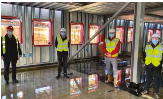
Ben Shenton, Acting Chair of Age Concern, with Andium Homes Chief Executive Ian K Gallichan and members of the project team on the site of the new facility. Works commenced in July 2020.
